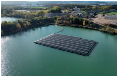
Arnstadt | 394 kWp | SolarEdge Technik
