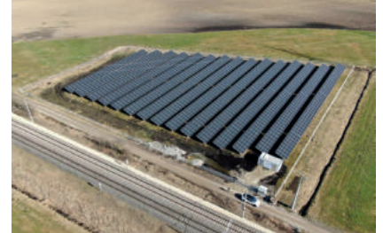
Bad Schussenried | 749 kWp
